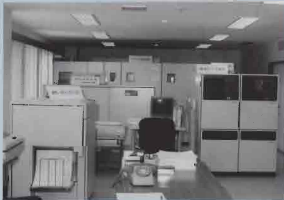
Computer room of NWEC
